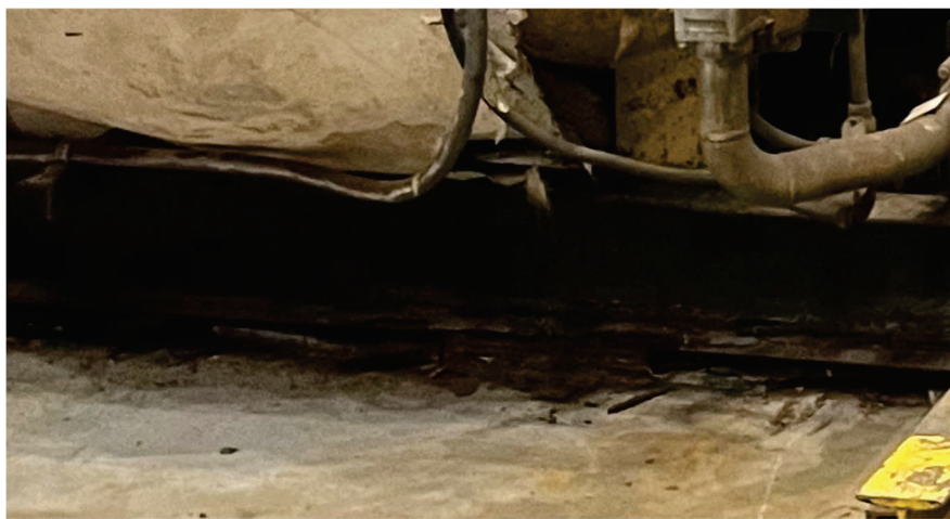
Photo 34B: Unit 1 Polisher Corrosion on Structural Supports
