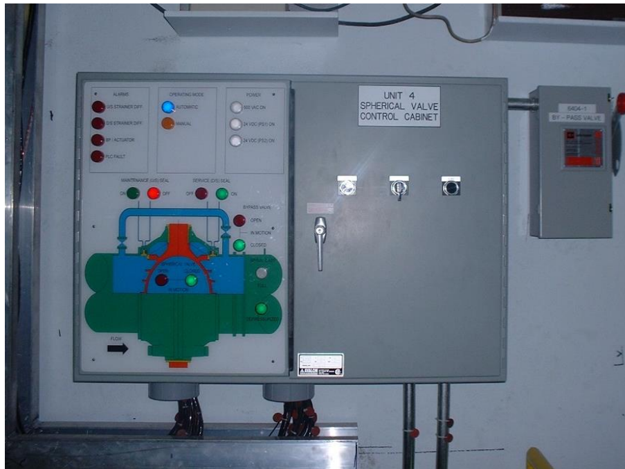
Figure 1: Spherical Valve Control Panel Exterior
