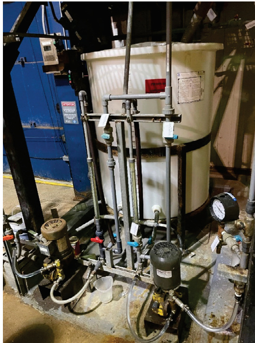
Photo 13: Coagulant Tank and Pumps
