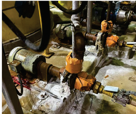
Photo 30: Caustic Transfer Pumps (2)
