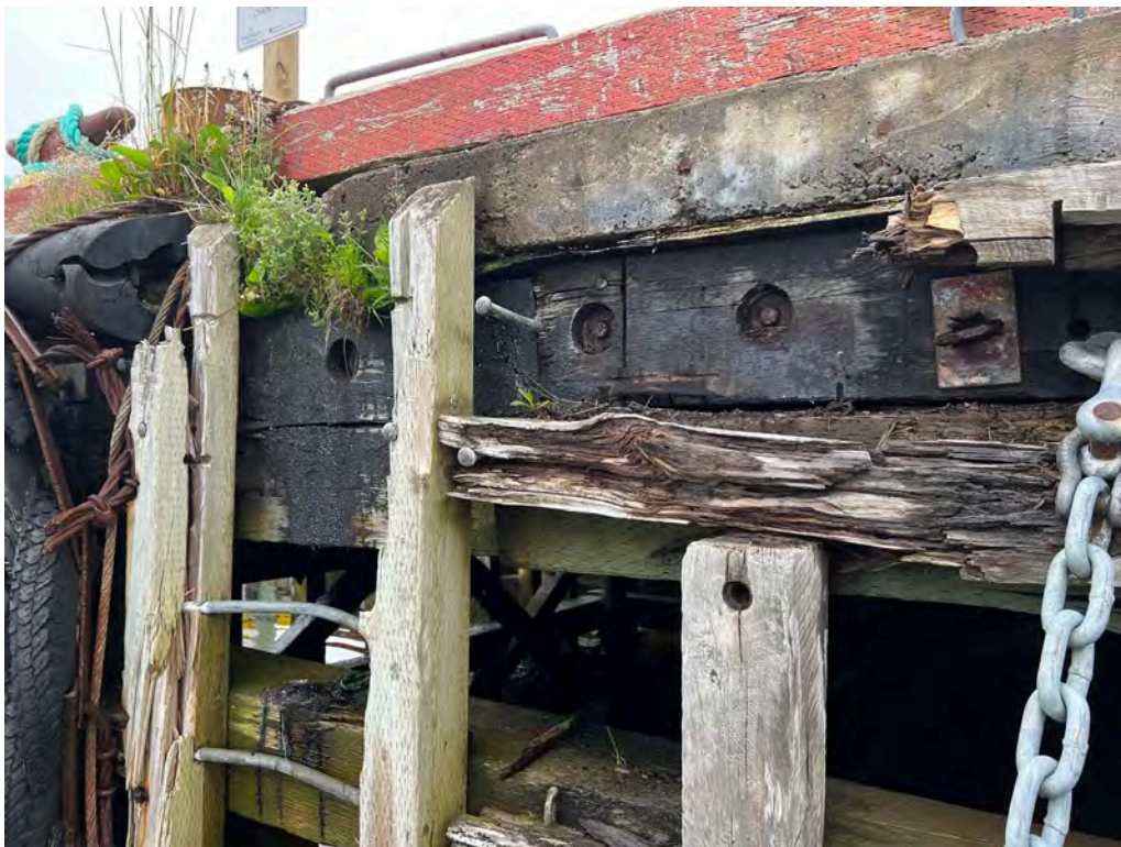
Poor condition of ladder, chocks and top rubber fender
