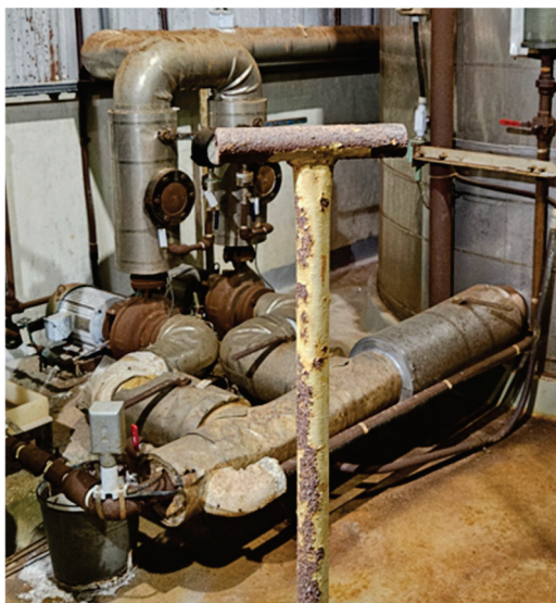
Photo 48: Caustic Transfer Pumps (2)
