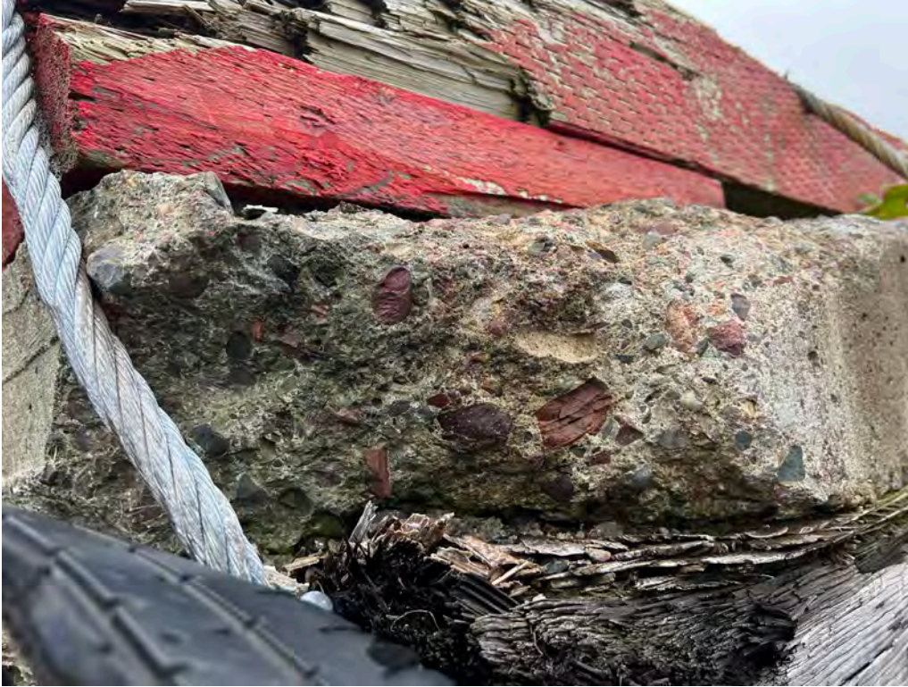
Concrete edge showing aggregate
