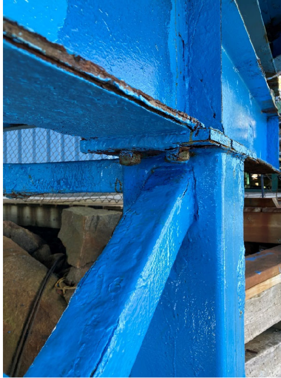
Photo 5: Corrosion along flange of beam
