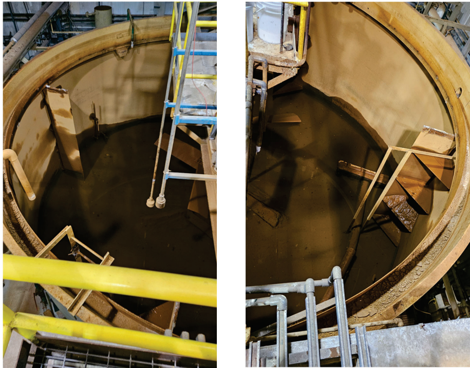
Photos 54 & 55: Batch Reactor
