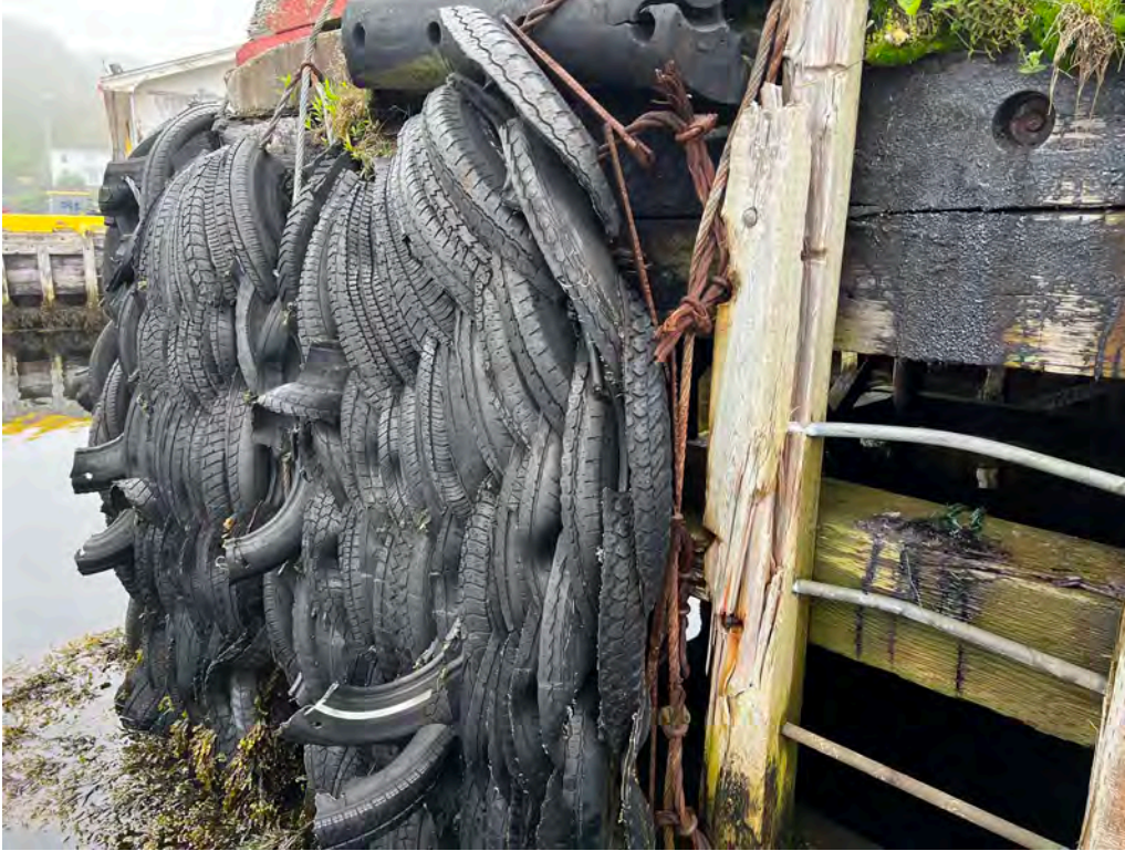
Corner blasting mat and poor condition of ladder
