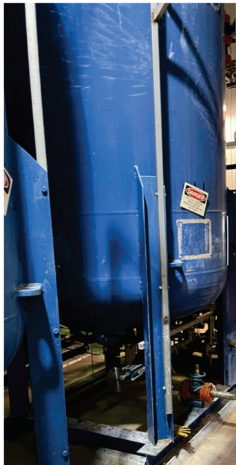
Photo 25: Anion Tank C (Cation Tank C in foreground)
