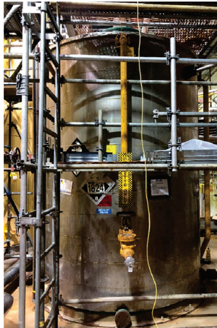
Photo 16: South 50% Caustic Tank (50%)
