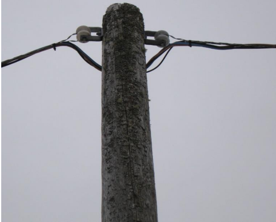
Figure 2: Example of a Deteriorated Pole
