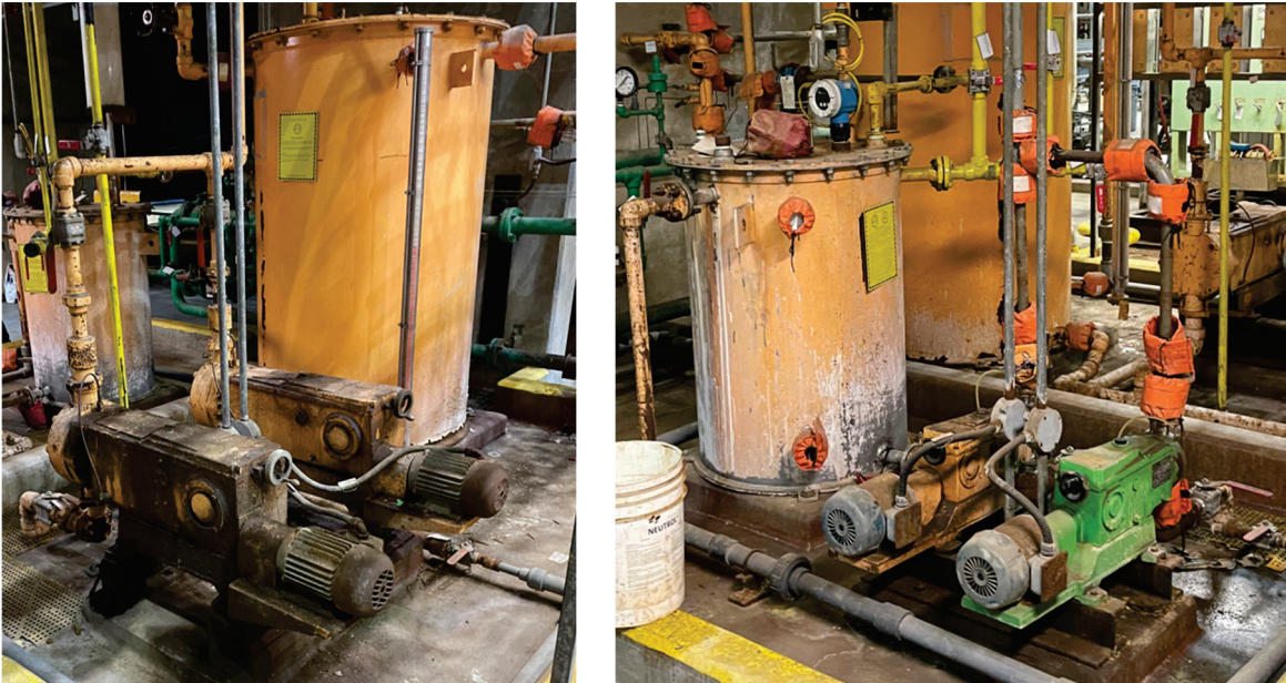
Photo 41 & 42: Unit 2 Caustic Transfer Pumps and Day Tank (left) and Acid Transfer Pumps and Day Tank (right)
