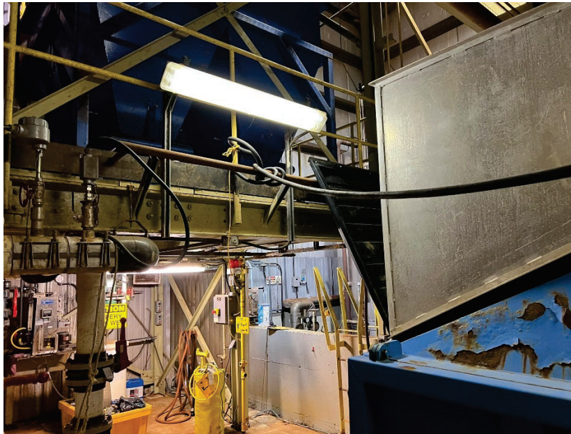
Photos 65: Cable routed haphazardly to unit heater
