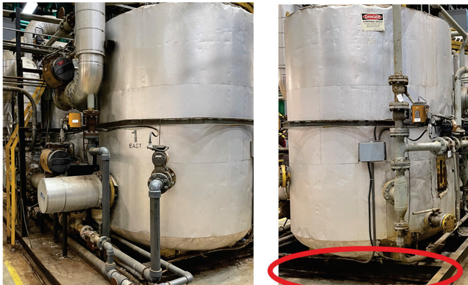
Photos 33 & 34A: Unit 1 Condensate Polishers
