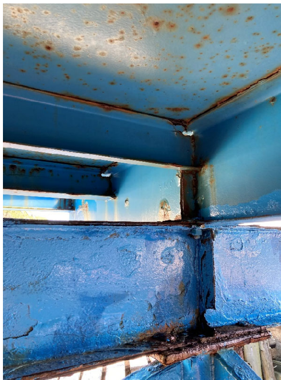
Photo 6: Corrosion beams and connections
