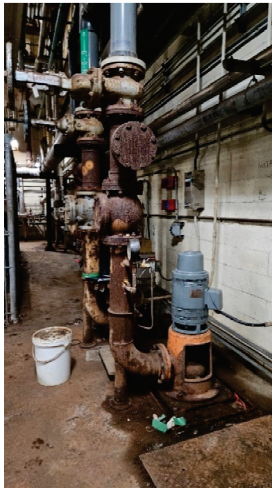
Photo 1: Raw Water Pumps
