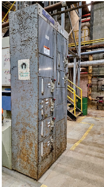
Photo 40A: Unit 2 MCC
