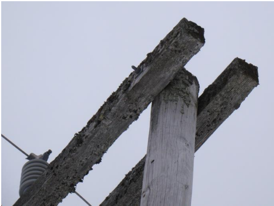
Figure 3: Example of a Deteriorated Crossarm
