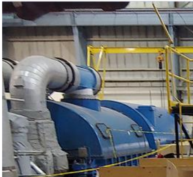
Figure 1: Holyrood TGS Unit 2 Turbine Generator
