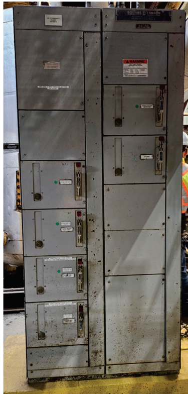
Photo 44A: Unit 3 MCC
