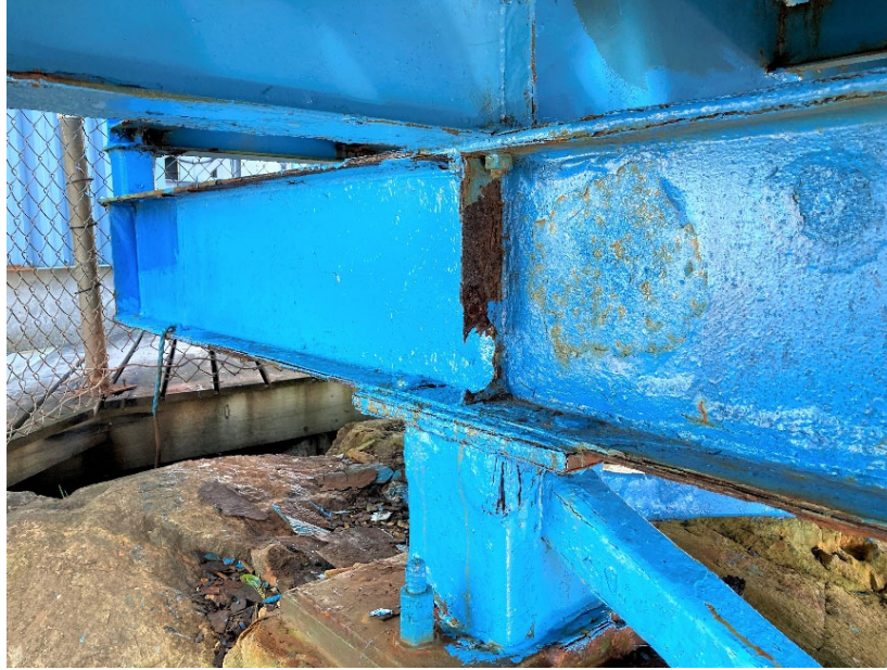
Photo 3: View along main support beam/corrosion through stiffener
