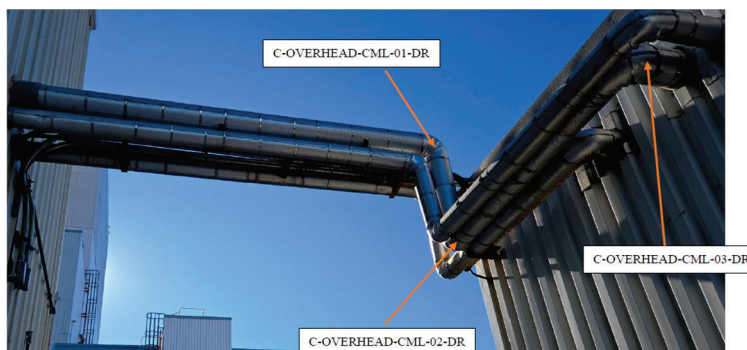
Photo 49: Overhead Caustic Piping (Exterior)
