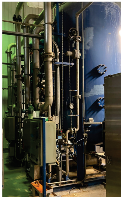
Photo 26: Mixed Bed Tanks (Edge of control panel in foreground)
