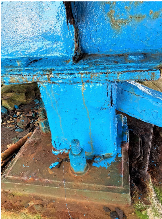
Photo 8: Loss in stiffener above column connection
