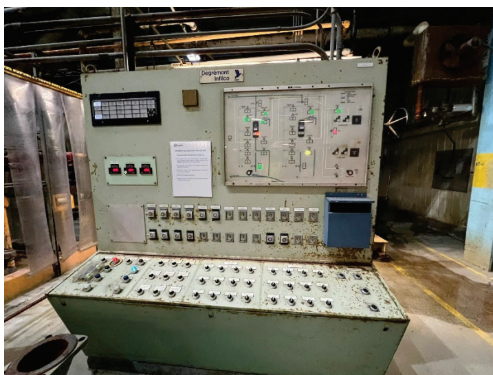
Photo 46: Unit 3 Control Panel
