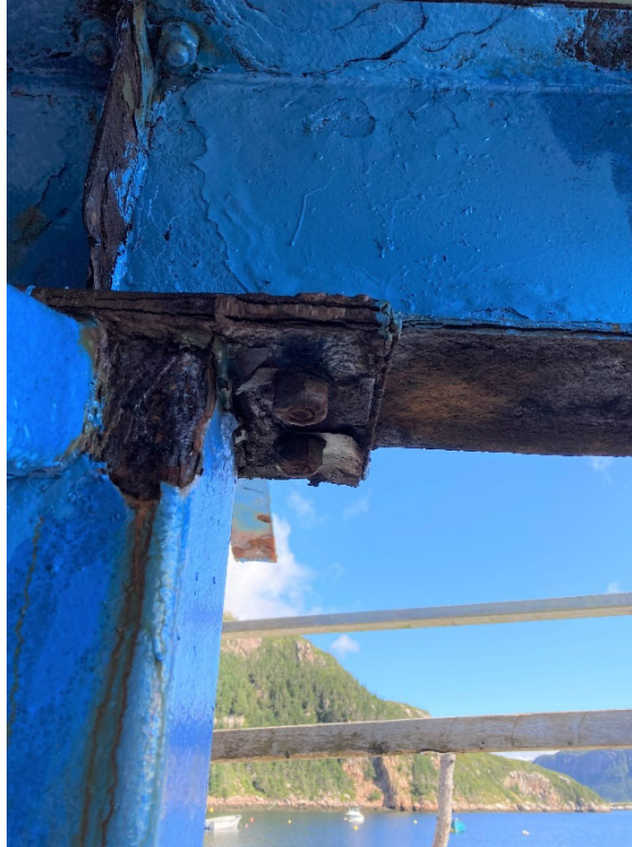
Photo 9: Corrosion at beam/column connection
