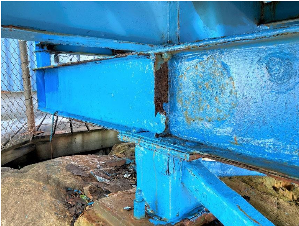
Figure 2: Corrosion through Stiffener on Main Support Beam
