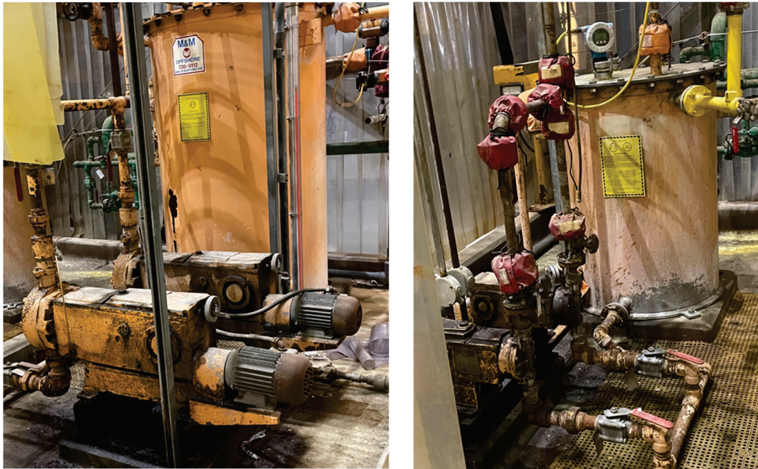
Photos 45A & 45B: Unit 3 Caustic Transfer Pumps and Day Tank (left) and Acid Transfer Pumps and Day Tank (right)
