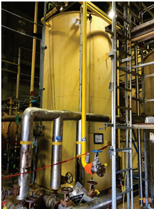
Photo 18: South Bulk Acid Storage Tank and Pumps
