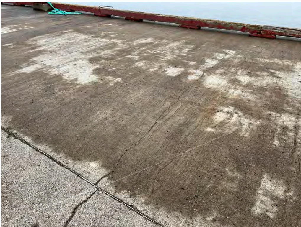
Transverse deck crack
