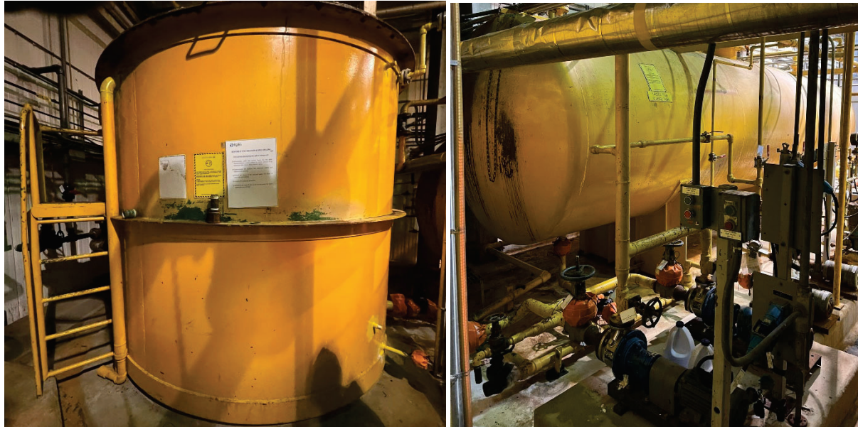
Photos 19 & 20: Melting Tank and Transfer Pumps
