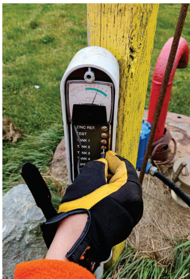
Photo 70: OWS No.2 Cathodic Protection Test
