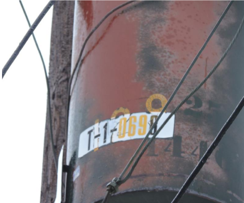
Figure 4: Example of a Deteriorated Transformer Tank
