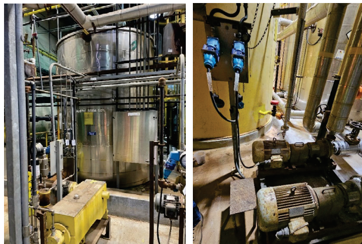
Photo 14 & 15: Caustic Tank (50%) and Pumps
