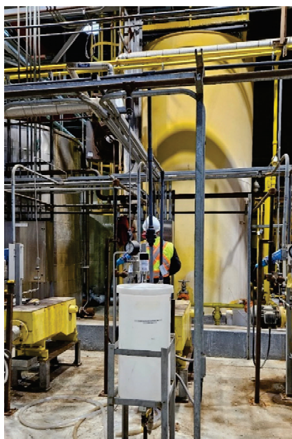
Photo 17: North Bulk Acid Storage Tank
