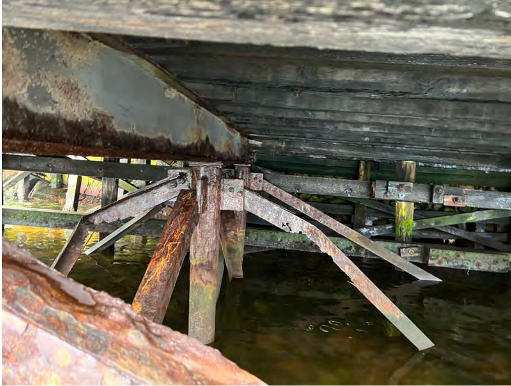
Poor condition of bracing
