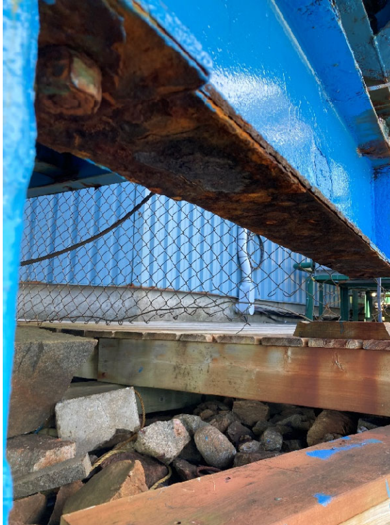
Photo 7: Corrosion at underside of beam
