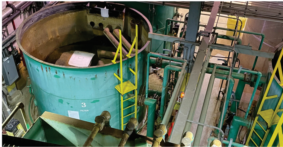
Photo 4C - Plan View of Sand Filter #3 (see piping from #1 & #2 routed through #3)
