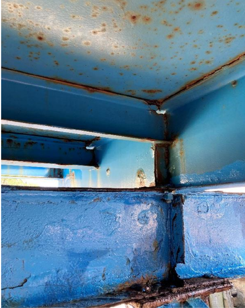
Figure 3: Corrosion of Beams and Connections
