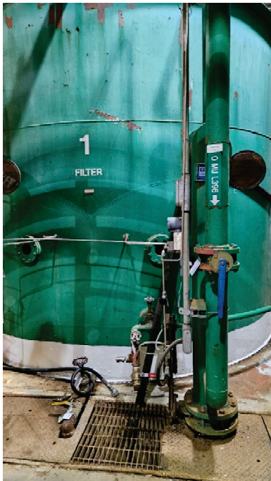
Photo 4A - Sand Filter #1 (typical)
