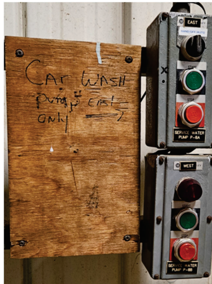
Photo 62: 'Makeshift' Control Panel for Pumps 8A/8B
