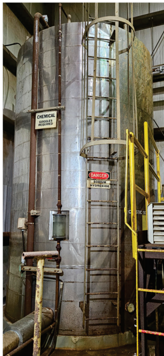
Photo 47: WWTP Caustic Tank
